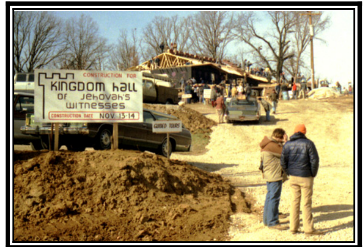
Jehovah's Witnesses from six surrounding states gathered to erect the new Festus, Mo., Kingdom Hall on Nov. 13-14.
